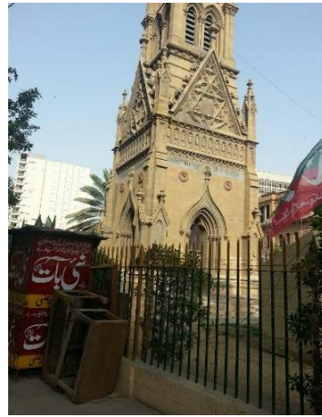
Fig. 12: Lack of Maintenance & Care.
