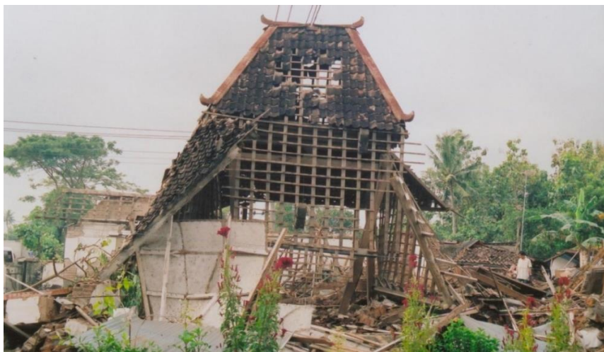
Fig. 2: A heavy damage joglo due to the 2006 earthquake: it but did not collapse completely; the core structure ( rong-rongan ) remains.
